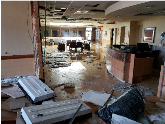
Damage after Hurricane Ida. This is often the state of disrepair that Soukup and his team encounter on assignments.
