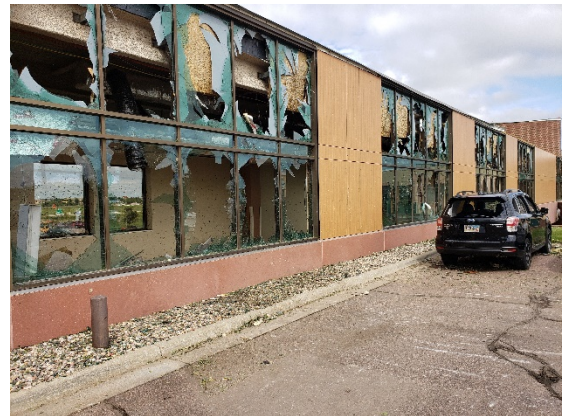
Blown out windows after Hurricane Ida
